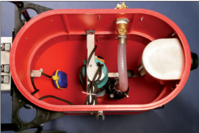
Inside view showing the pump and the float switch for the suction motor and pump.
